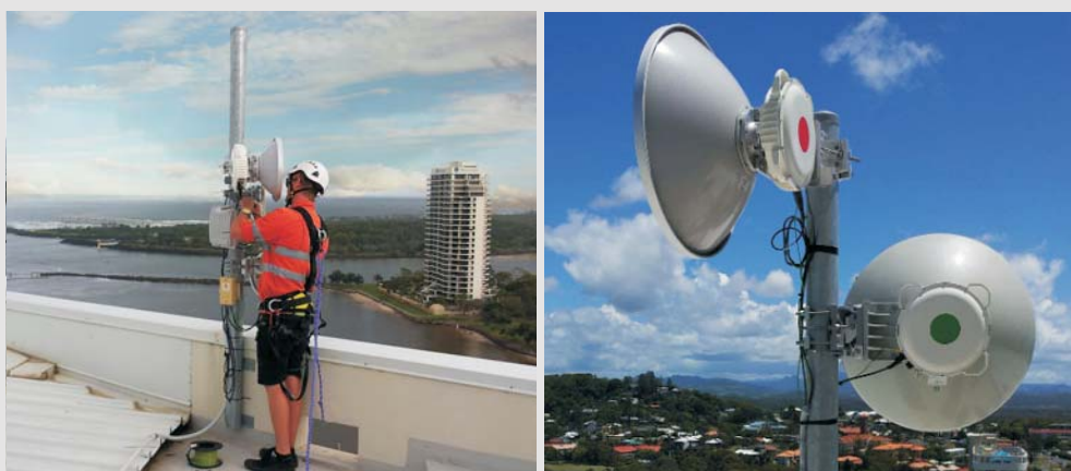
Installation of SAF Microwave Radios for Twin Towns Clubs & Resorts by Wires Networks (subsidiary of Wires Broadband- World Without Wires)
