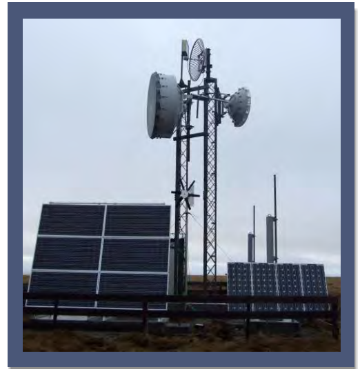
■ Solar powered CFQ site
